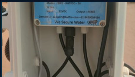
RTU & CHARGE CONTROLLER
